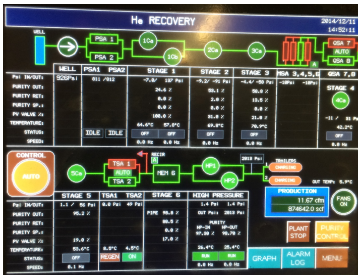
HMI for the first Quantum production plant – plant runs essentially unmanned
