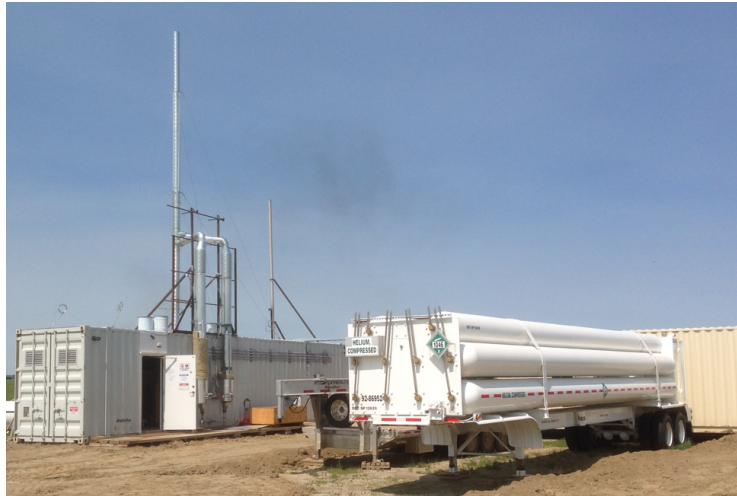
Quantum Plant in Saskatchewan, first production plant in Canada in 40 years, started in 2014
