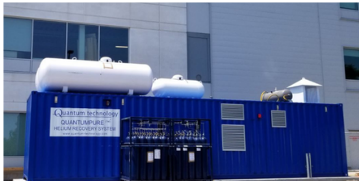
Helium Recovery and Nitrogen Generation System at North Eastern University
